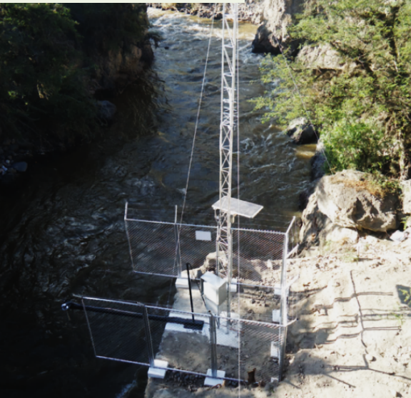
Automatic Weather Station (AWS)
